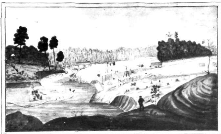
Brewers Lower Mill; excavations of canal and construction of locks in progress; note the barrow run on the left side of the picture; Burrowes Sketch, Archives of Ontario
