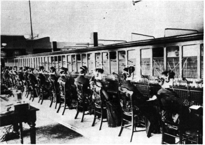
First multiple switchboard in Montreal installed in the British Empire Assurance Company Building, April 1886. At that period, all the operating labour force in big exchanges was constituted of women. (Photo #3109 Courtesy of Bell Canada Telephone Historical Collection)
