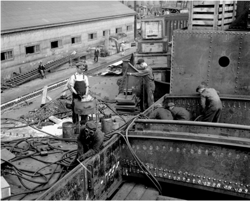
Men at work on a 10,000-ton dry cargo ship in a Montreal shipyard. Note the burner at left operating an oxy-acetylene torch. Behind him standing on deck is a heater with his portable furnace for heating rivets. At the right a group of workers include a riveter and a holder on.
