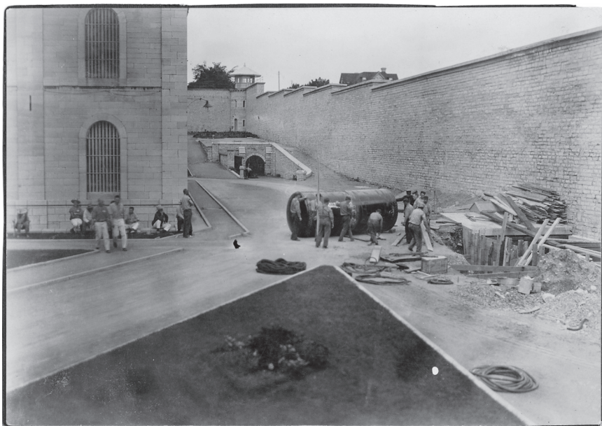
Kingston Penitentiary, 25 October 1933. The prisoners on the left are taking their break outside the south face of the prison hospital, while on the right an excavation team prepares to install a new oil drum.
